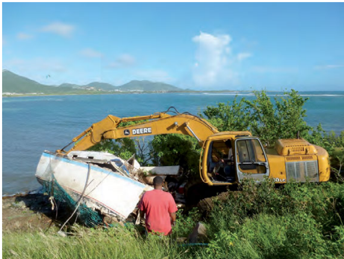
Beau travail de la pelle mécanique A hard work by the mechanical shovel
